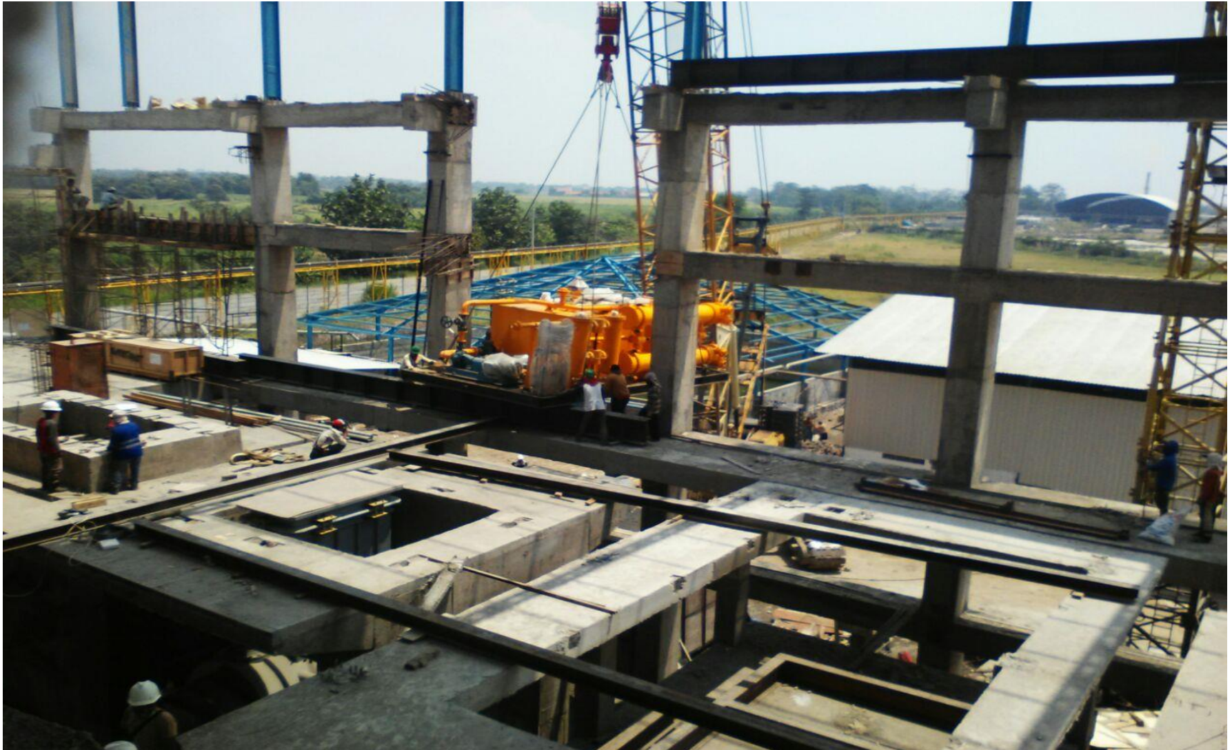
Lifting Lube Oil System for Steam Turbine Unit # 1
